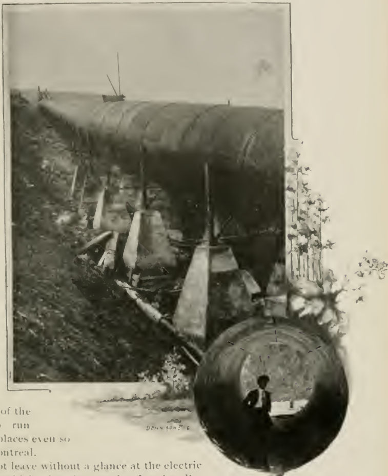
One of the Big Penstocks
